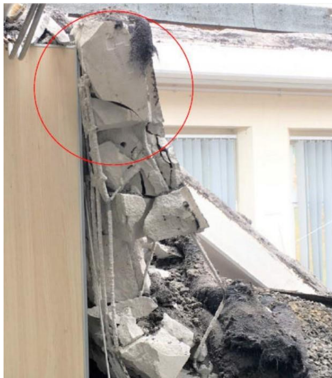
Figure 2: 2018 Roof Slab Collapsing (SCOSS)
